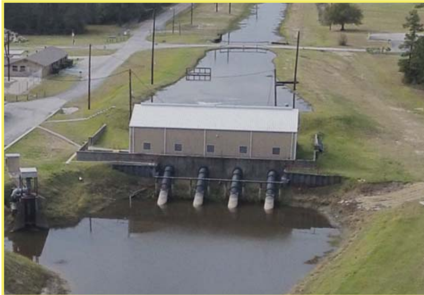
Gulf Coast Division Pumping Plant
