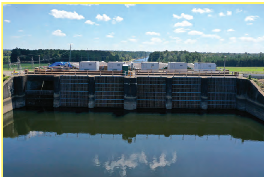
Toledo Bend Powerhouse, New Forebay Trash Racks
