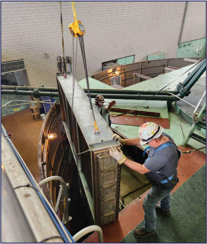
Powerhouse Unit #2 outage
