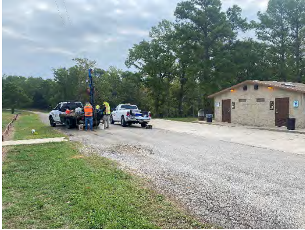
Distressed Pavement Near Boring B-04
