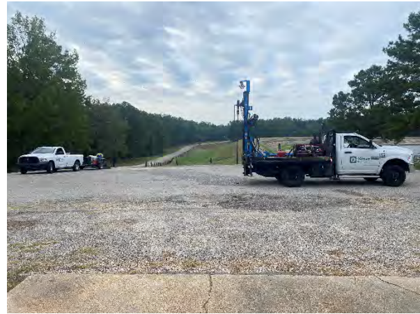
Distressed Pavement Near Boring B-02
