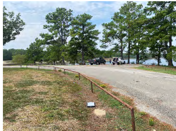
Distressed Pavement Near Boring B-03
