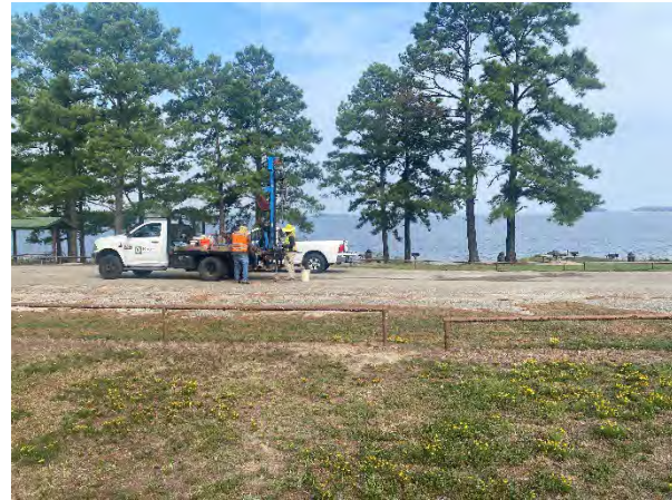
Distressed Pavement Near Boring B-07
