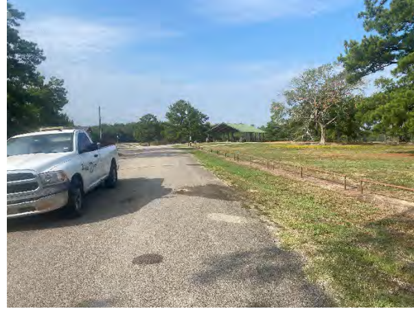
Longitudinal Crack Near Boring B-05
