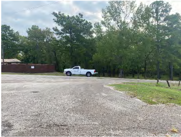
Distressed Pavement Near Boring B-01
