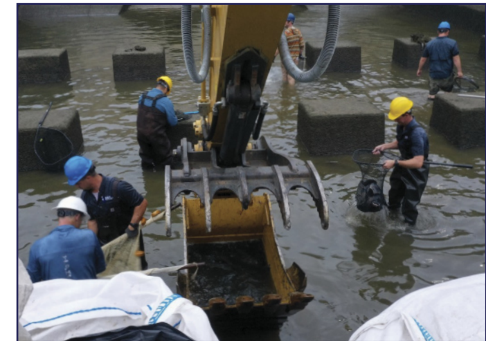
Relocating fish from the Tawakoni Spillway to the downstream side of a cofferdam
