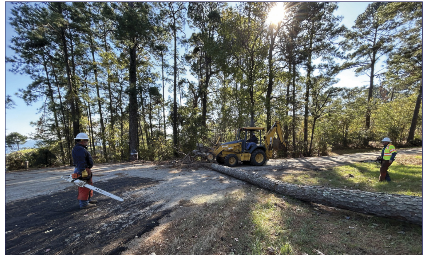
Tree hazard removal at East Hamilton Recreation Area
